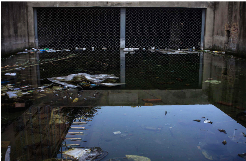
Drowning: The flooded underground parking lot at the historical landmark helps tip the condition of the historic square from one of mere neglect into actual squalor.
